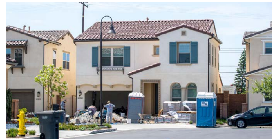
A home under construction on Elizabeth Lane in Buena Park, on Thursday, July 12, 2018, the former site of Dickerson Elementary School which is now a residential neighborhood.
